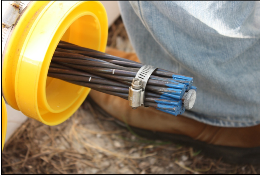
Figure 6 Strand Group Ready for Duct Insertion with Galvanized Spike Secured with Stainless Steel Hose Clamp
