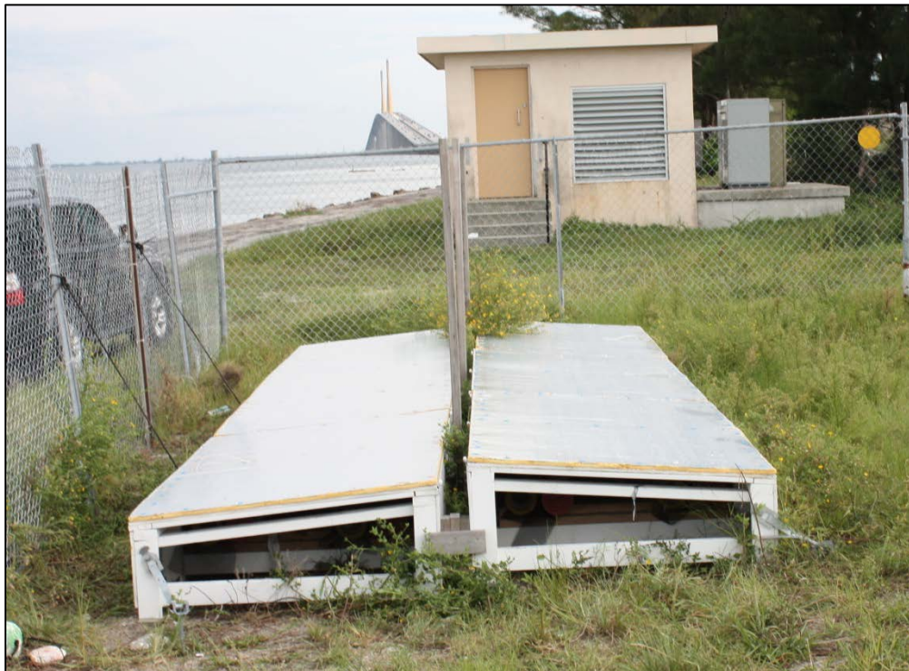
Figure 3 SSK Duct Facility in the Closed Position - Sunshine Skyway Bridge Main Span and Generator Control Room in the Background
