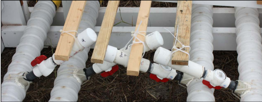
Figure 4 Relative Humidity & Temperature Probe Housings Attached to Ducts via Vent Port and Secured with Wood Boards and Zip-Ties
