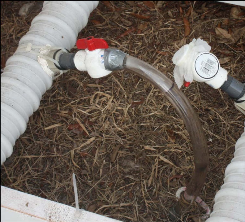
Figure 5 Water Reservoir Attached via Vent Port (left) and Closed Vent Port Covered with Bug Shield (Right)
